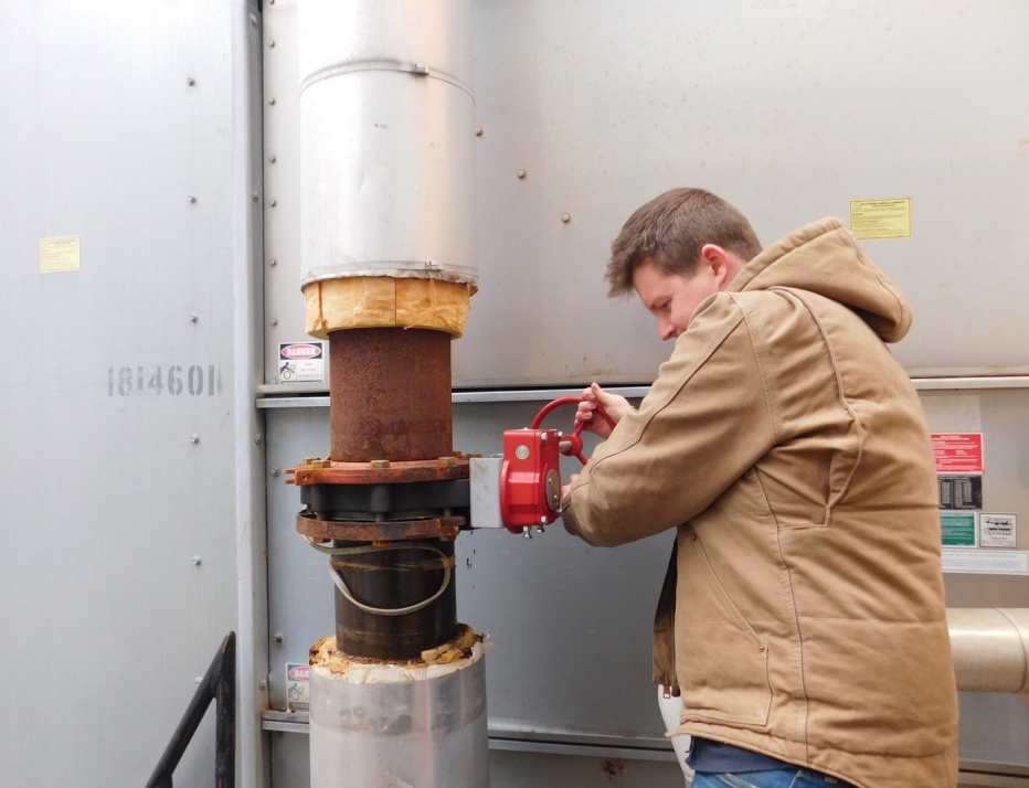
Photographed Above: Michael Brusic, Technical Director at Bright Power, testing out the new cooling tower isolation valves.
